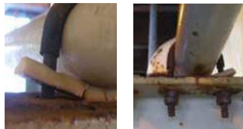
Failed I-Rod® imitations.
